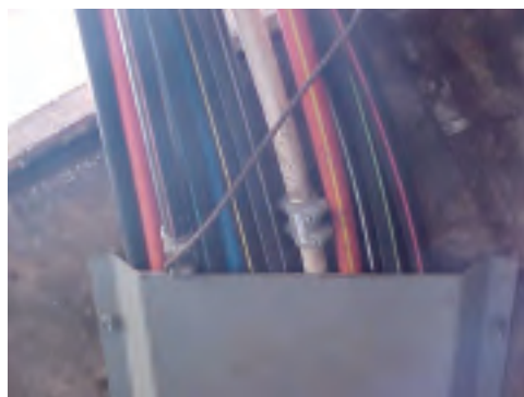
LSZH conduit entering tunnel into metallic tray.
